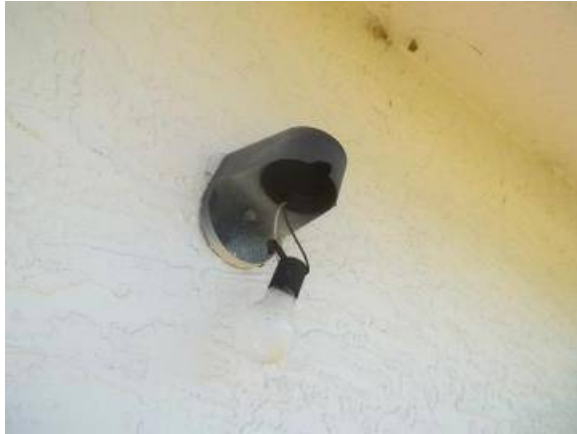
Exterior light fixture hanging from wires near the pedestrian door.
