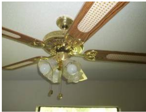
Ceiling fan in the left of the hall bedroom is not operating.
