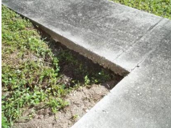
Uncontrolled rain water from the roof has caused undermining of the sidewalk.
